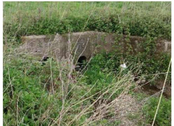
Figure 3-10 Farm Access Culvert 2 Outlet
