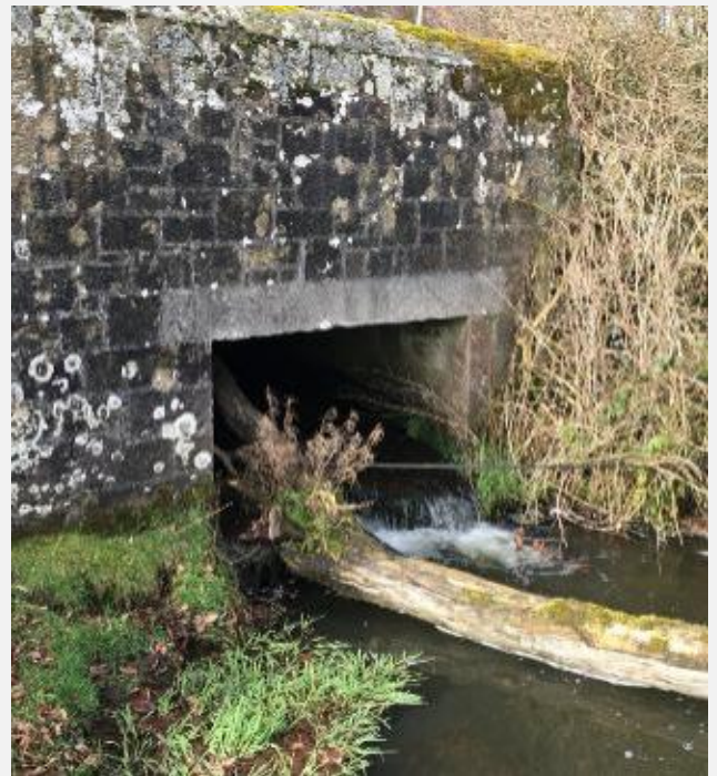
Figure 3-31 Shipperton Bridge (Outlet)
