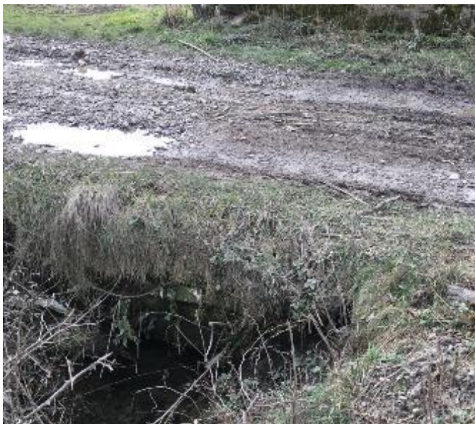
Figure 3-26 Tributary of Embleton Burn culvert (outlet)
