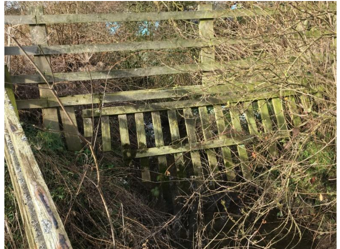
Figure 3-24 Debris Fence along Unnamed Western Tributary of Kittycarter Burn
